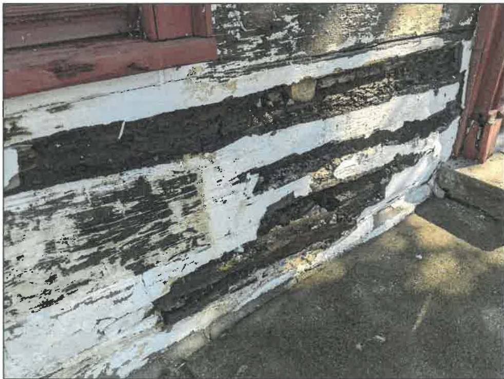
Detail of damage to logs on the south elevation caused by rot and insects.
