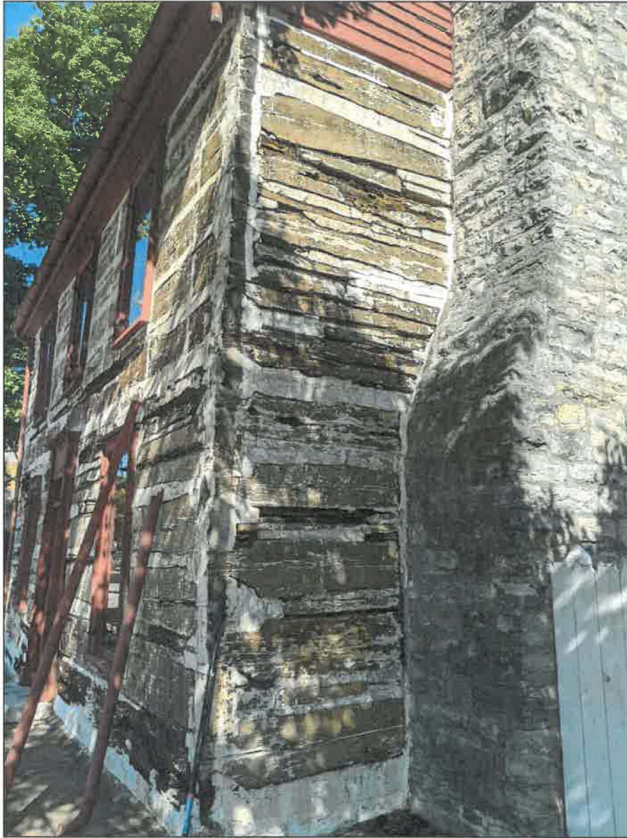
View of the east elevation caused by rot and insects.
